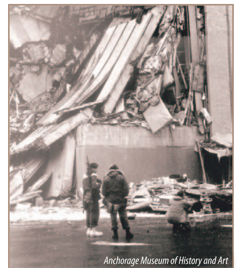
The J.C. Penny building in downtown Anchorage was heavily damaged during the 1964 Good Friday earthquake.
