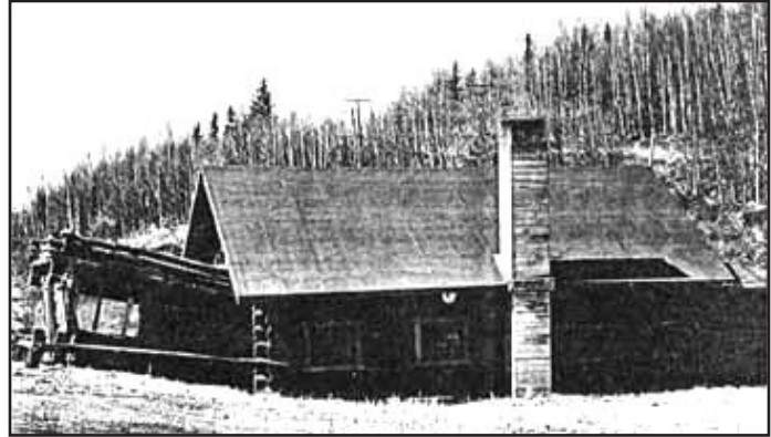
Photo courtesy of CRREL, the U.S. Army corps of Engineers, printed in the July 20, 1984 edition of the Alaska Science Forum, Coping with the Permafrost Foundation.
