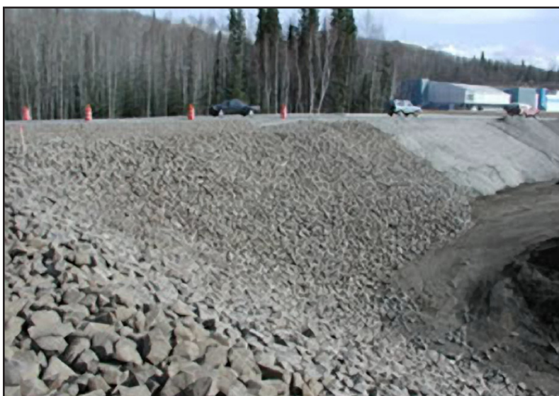
Air convection embankment on Thompson Drive at the University of Alaska Fairbanks. Photo courtesy of the University of Alaska Fairbanks Mechanical Engineering Department.
