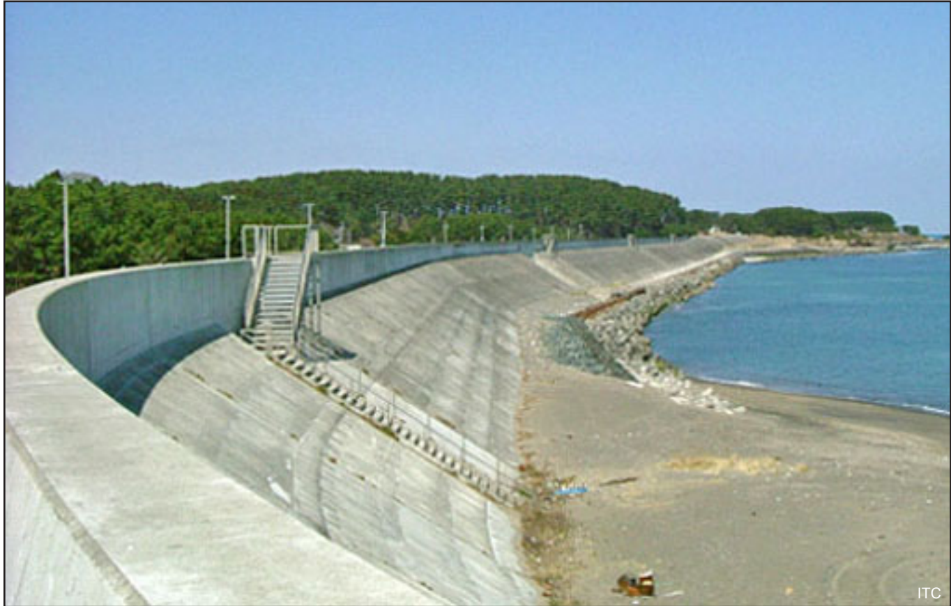
Sea wall with stairway evacuation route used to protect a coastal town against tsunami inundation in Japan. Photo courtesy of River Bureau, Ministry of Land, Infrastructure and Transport, Japan.
